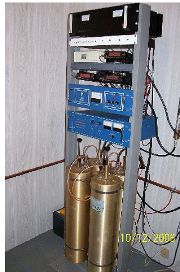
Repeater and Remotes
