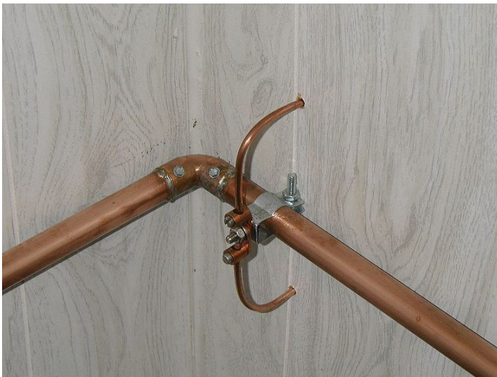
Part of the Grounding System
